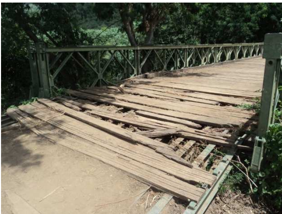
Picha 2 The damage is now affecting the steel frames
